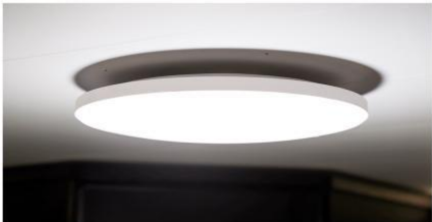
Ceiling Lights Bright & well-lit interior
